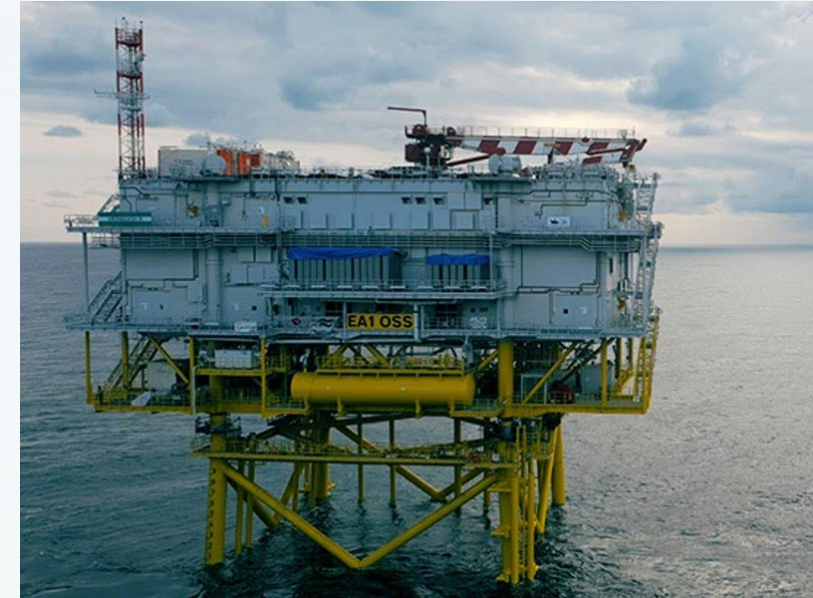
HVAC substation (714MW)
