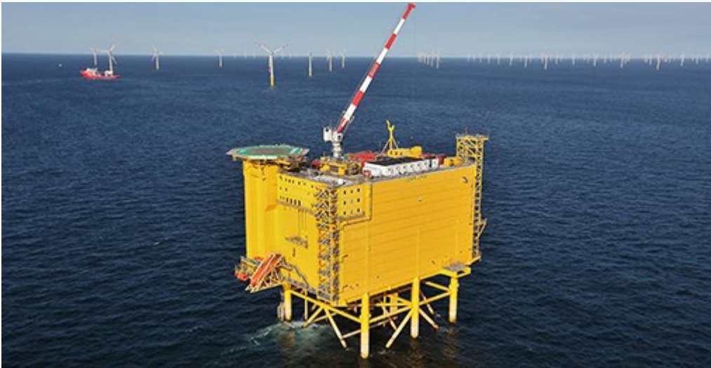
HVDC convertor station (800MW)
